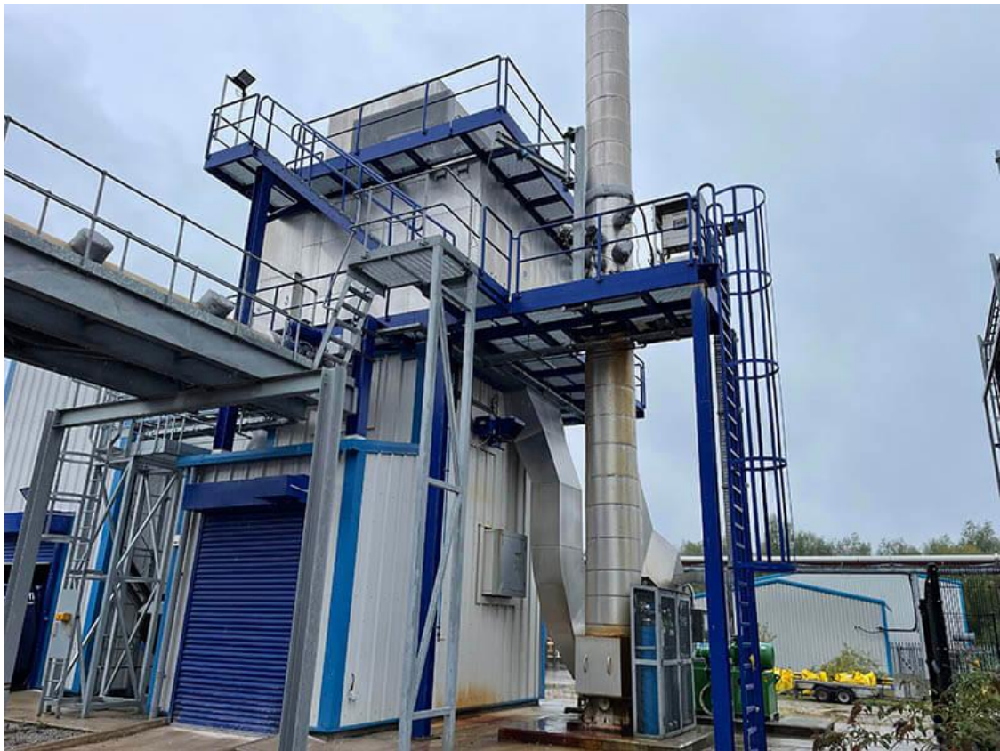
Glass Fibre Furnace Abatement Plant - Lancashire
