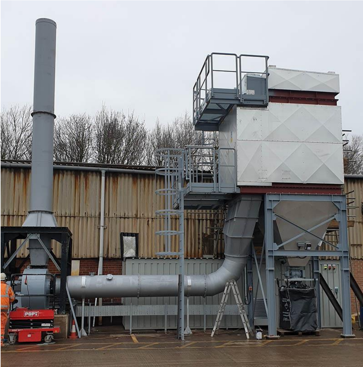
Galvanising Plant Filter - South Wales
