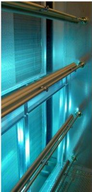
Multiple Coil-clean units in operation
